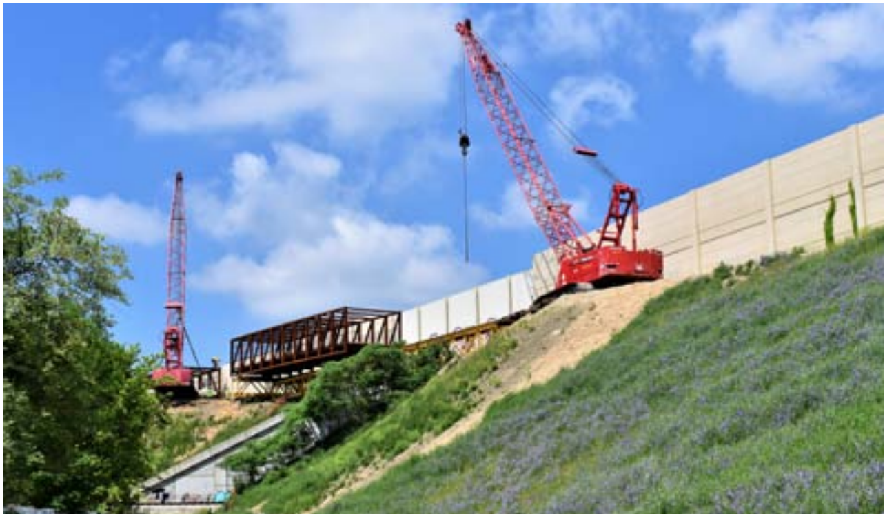
In 2018, the central link in the Fred Meijer M-6 Trail was completed with two new bridges and a mile of newly paved trail.
